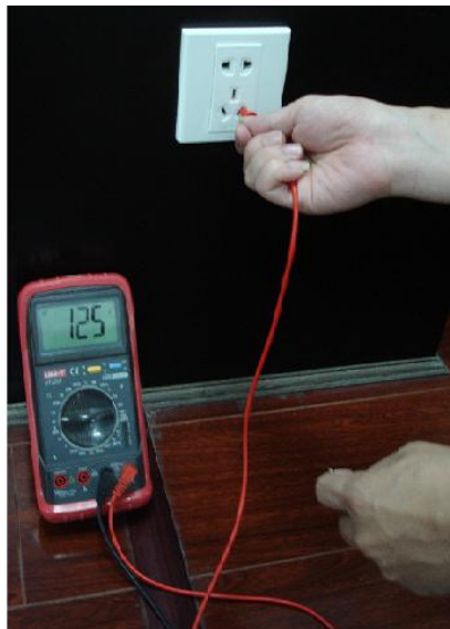
Appendix Figure 7-6 Check live cable connection
